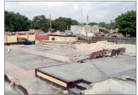
A concrete pad is all that remains of the Haiti Ministries church in Port-au-Prince.
