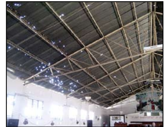
Harmony Church #1 in Port au Prince has holes in its sanctuary roof from gunfire between U.N. soldiers and gangs from 2006. No one was in the church at the time of the fighting.
